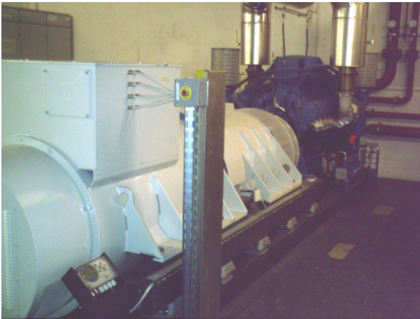
Figure 2 Genset 720kVA / 640 kW with rotating energy storage
